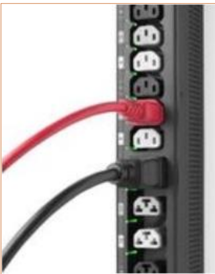
A C14 and C20 Plug Connected to Cx Outlets
